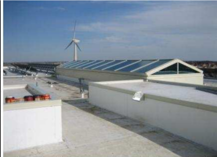
A white roof and daylight atrium harvest daylight and reduce the energy needed for lighting.
