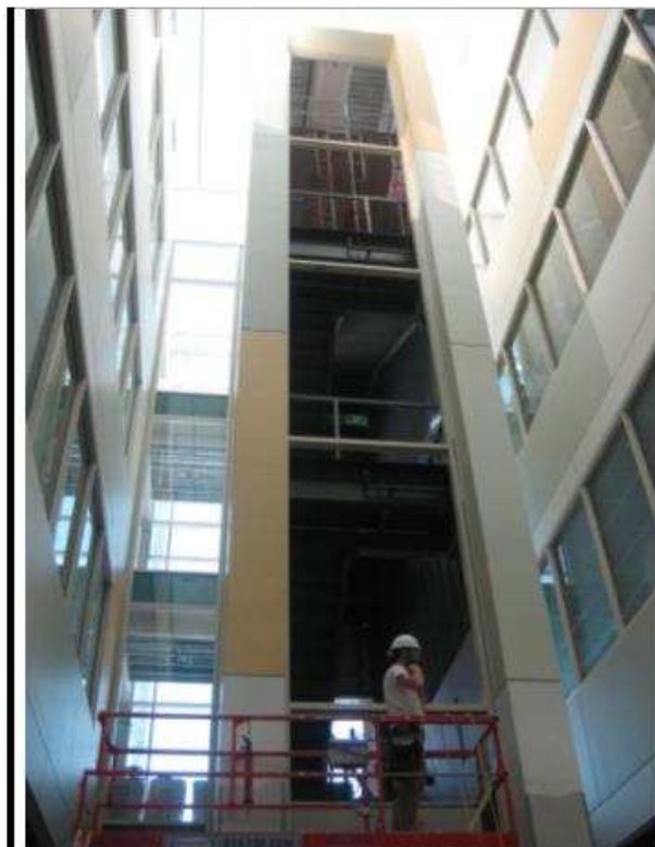
The daylighting atriums served as a light source even while construction was still underway.
