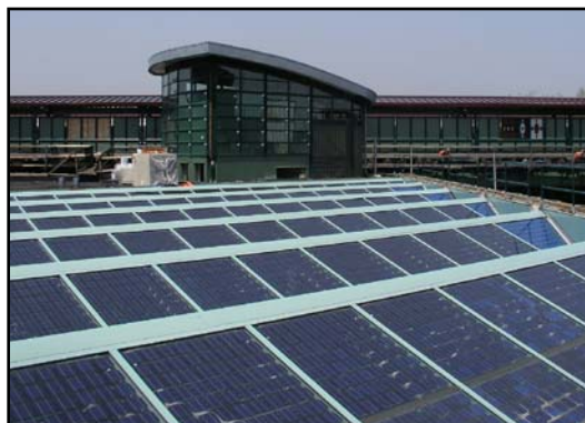
Solar Panels on Roof of New York City Transit Roosevelt Avenue -74th St. Station
